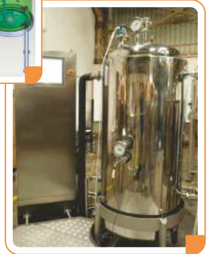
Pressurized Hot Water Tank (350 Ltr)
